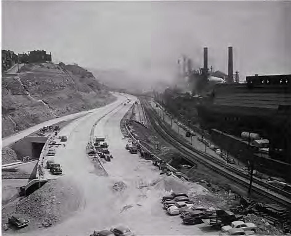
Fig. 5. Hare, Clyde. Penn-Lincoln Parkway Construction . 1951. Carnegie Museum of Art Collection of Photographs. Accessed: https://historicpittsburgh.org/islandora/object/pitt%3A86.16.93
