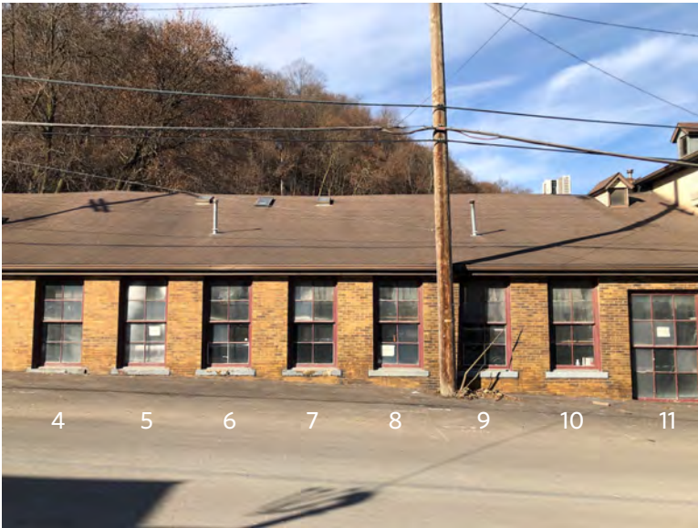
Photo 11. South facade, looking north, showing Bays 4 through 11 in the shed portion of the building.
