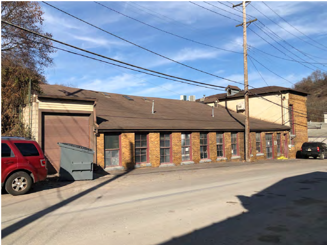
Photo 9. South facade, looking northeast, showing the entrance into the garage/loading dock in the first bay of the shed.
