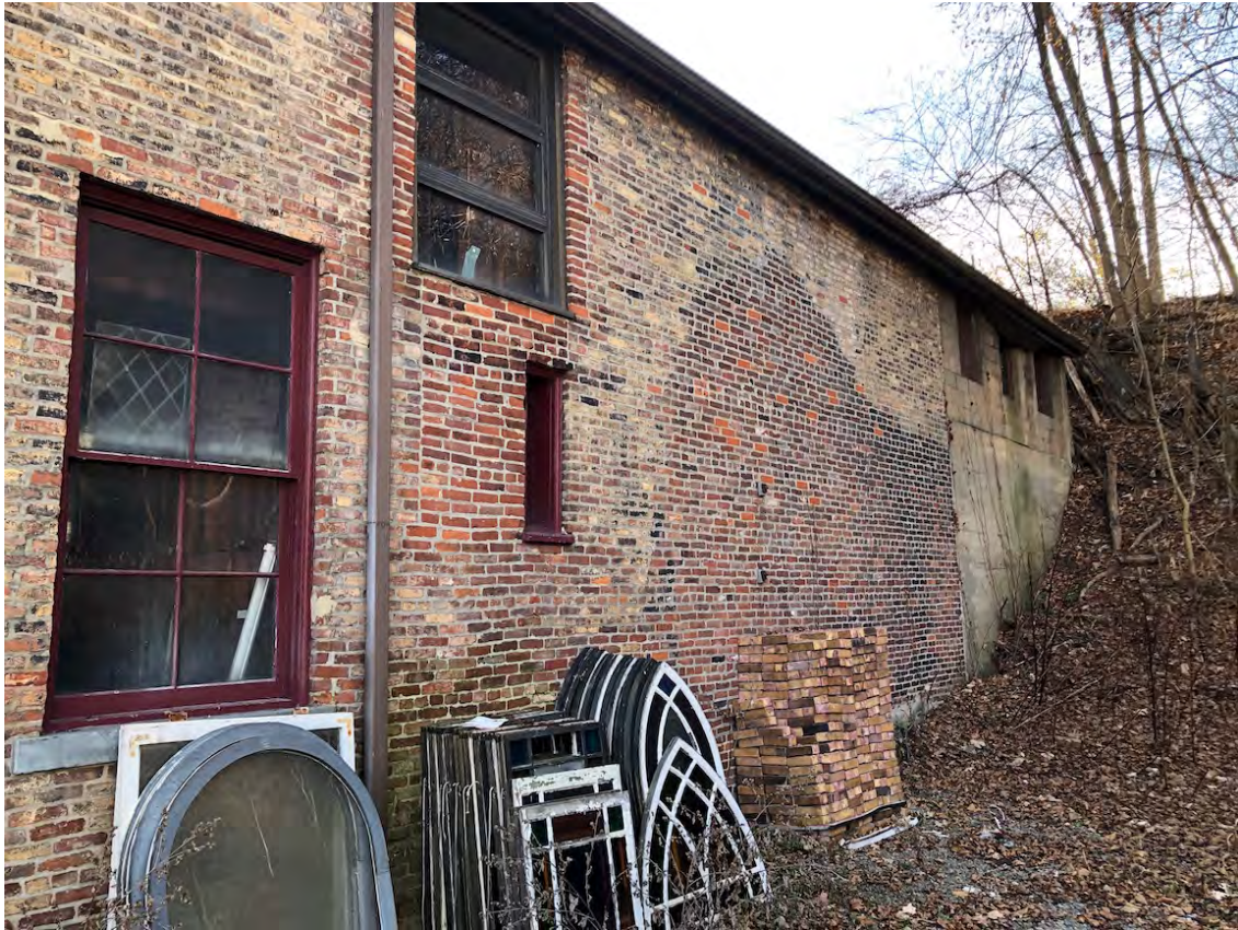
Photo 15. Rear half of the north facade, looking southwest, showing Bays 5 and 6 of the shed (left) and the 1946 concrete block addition (far right).
