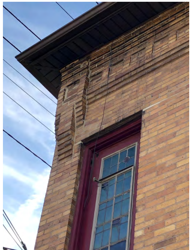
Photo 7. Detail, front facade, looking southwest, showing the decorative brick cornice above a leaded window.
