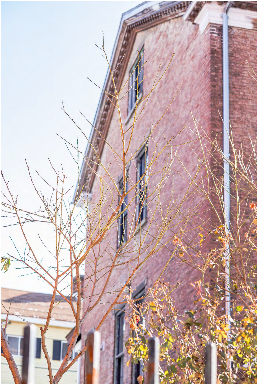
Photo. 4. Echo, Cornice Detail , January 10, 2020. Source: Preservation Pittsburgh.
