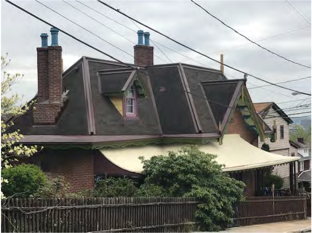
Photo. 12. Heathside Cottage, SSE Myler Street, Roof Detail, April 2019. Source: Matthew W.C. Falcone.
