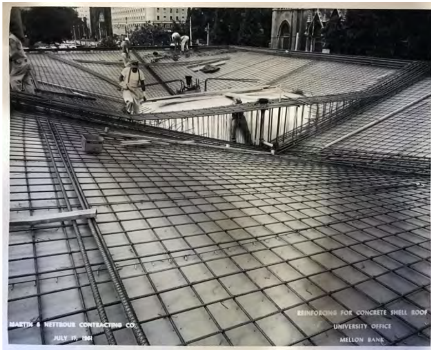
Figure 28/29: University Office under construction showing Top: erection of thin-shell concrete form. Bot: rebar layout. July 1961. Heinz History Center, Mellon Bank Records. Demolished 2004.
