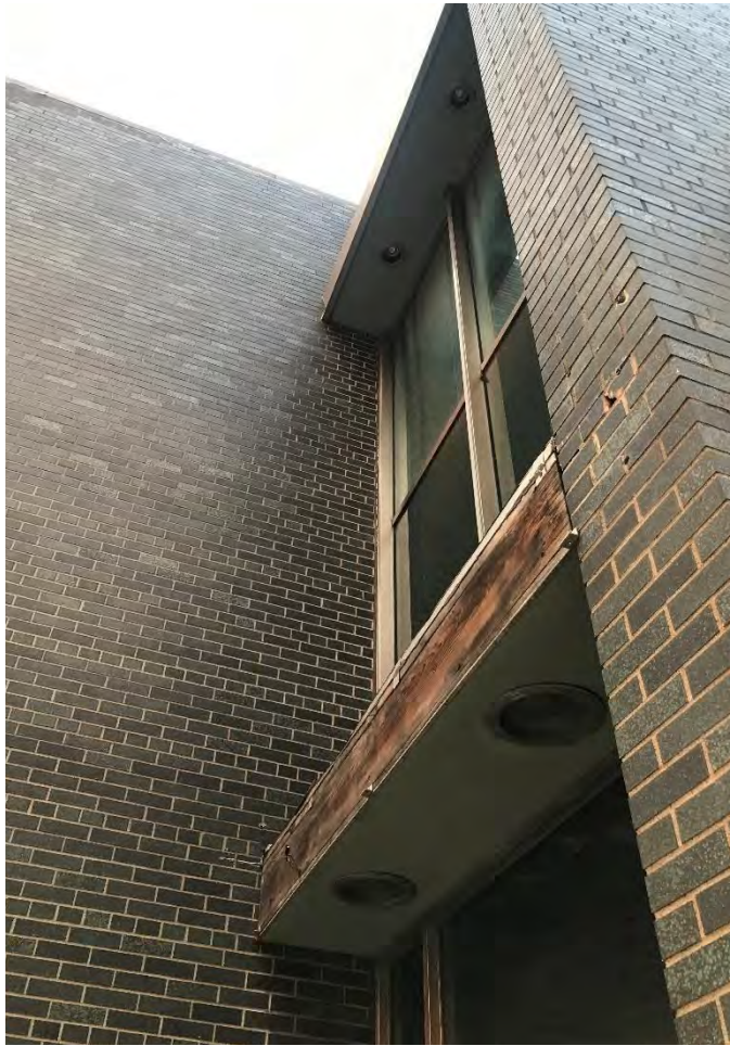
Figure 10: Mellon National Bank, East Liberty Office, detail view showing wall and glazing juncture on southwest (rear) facade, facing northwest (Brittany Reilly).
