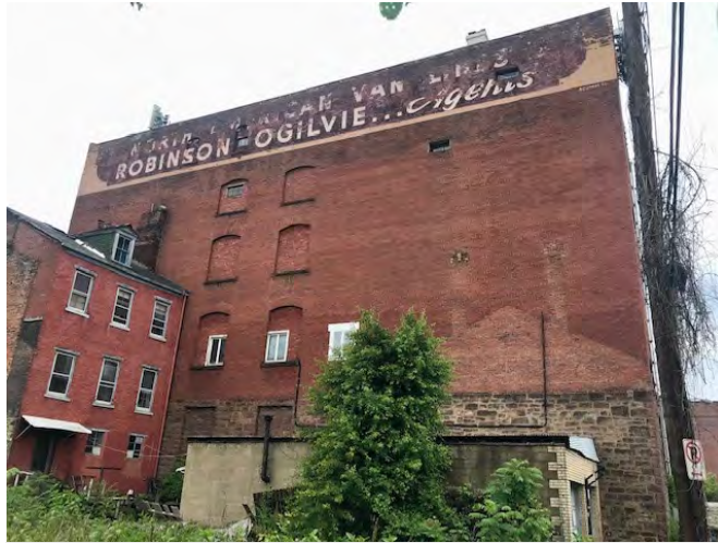
Photo. 6. West Tertiary Façade, 855 S. Canal Street. Matthew Falcone. May 2023.
